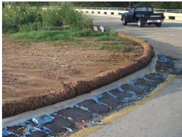
After rain the next day. Note how clean the road is - and the sediment is behind the EcoWattles.
